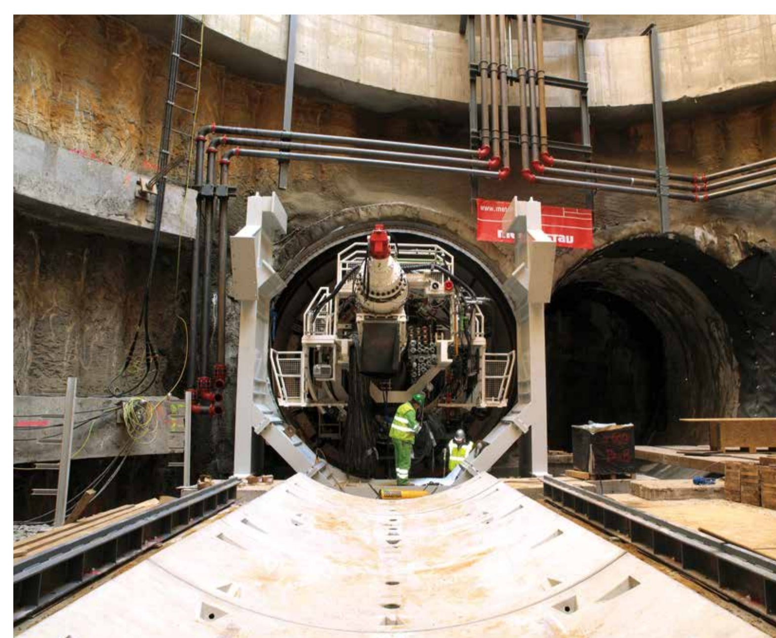
Instalace razičeho štítu v pažené jámě – prodloužení metra A – archiv Metrostav, Praha Installation of the TBM (tunnelling boring machine) in a sheeted foundation pit – extension of the Metro line A – Metrostav Co. archives, Prague, the Czech Republic
