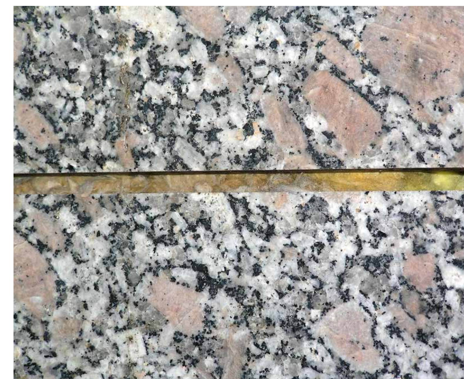
Tepelná izolace fasády za obkladem v ohrožení vodou – Archiv hl. m. Prahy Façade thermal insulation behind the stone veneer endangered by leaking water – The Prague City Archives, the Czech Republic
