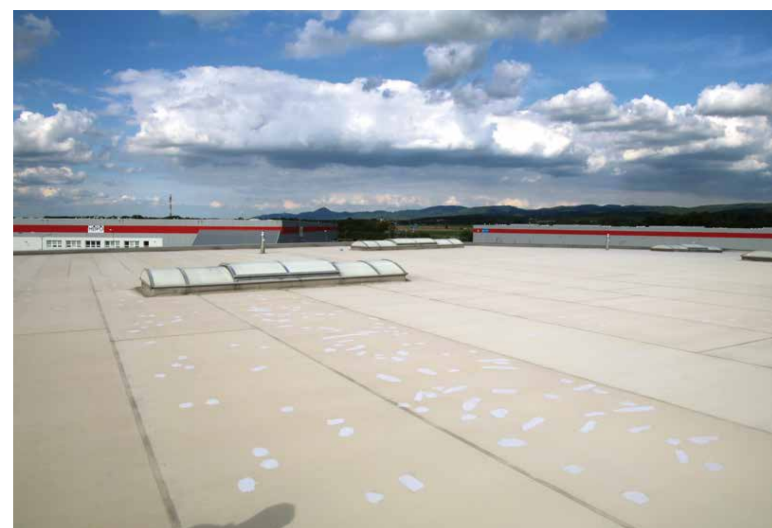
Celkový pohled na střechu poničenou kroupami – snaha o opravu nátěrem byla naprosto neúspěšná General picture of a roof damaged by hail – the effort to repair the roof by a coat of paint was absolutely fruitless.
