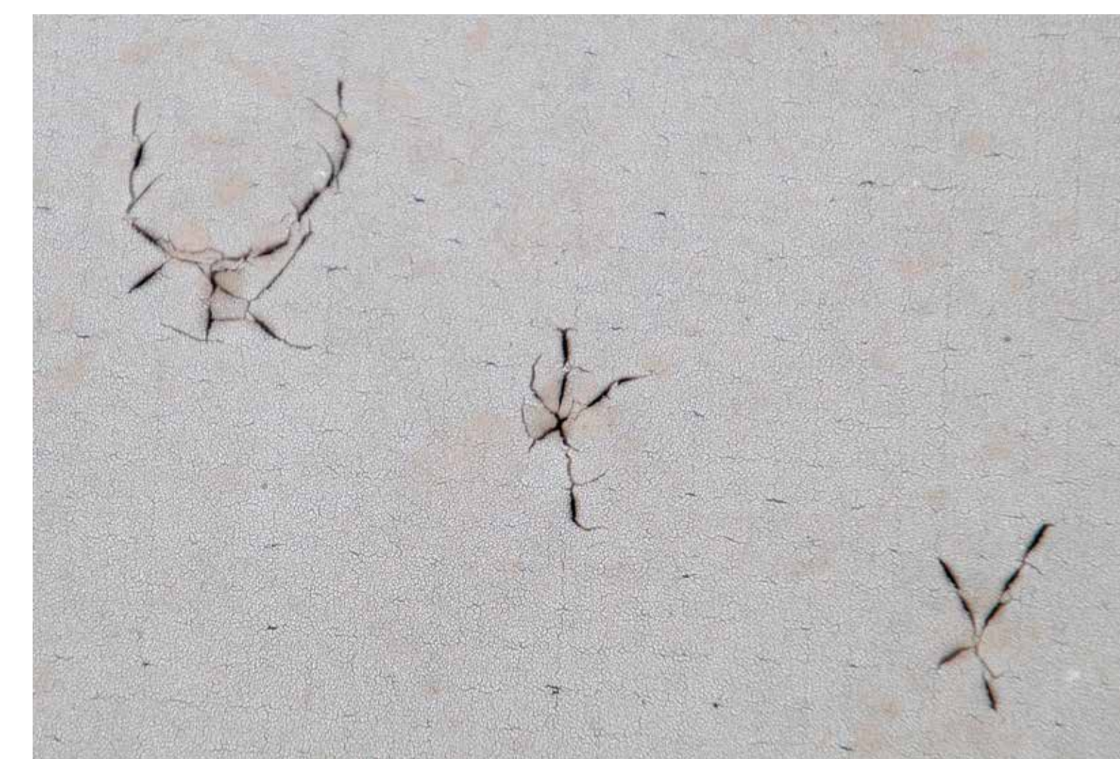
Poničení fóliové hydroizolace kroupami (detail) Foil damp proof course damaged by hail (detail)
